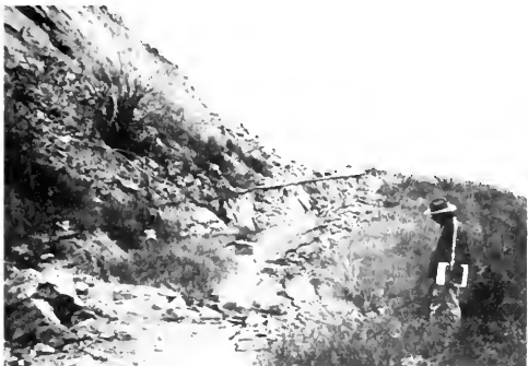
Photo 10. Earthquake-caused damage to a minor road on the east side of Indian Canyon 490 m (1600 feet) northeast of Oak Hill School. The landslide and rockfalls are both related to the failure of dip slopes in Towsley/Pico sandstone and conglomerate beds. Bedding planes are visible in the upper left portion of the photo.
